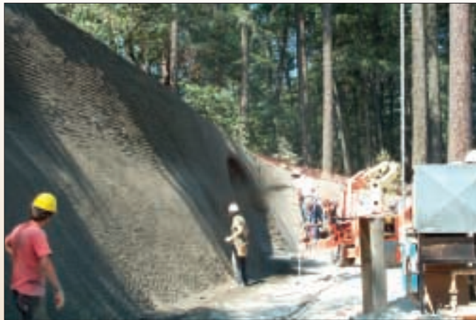
At the portals, soil nail and shotcrete walls are typically used for permanent support and are constructed from the top down in lifts.
