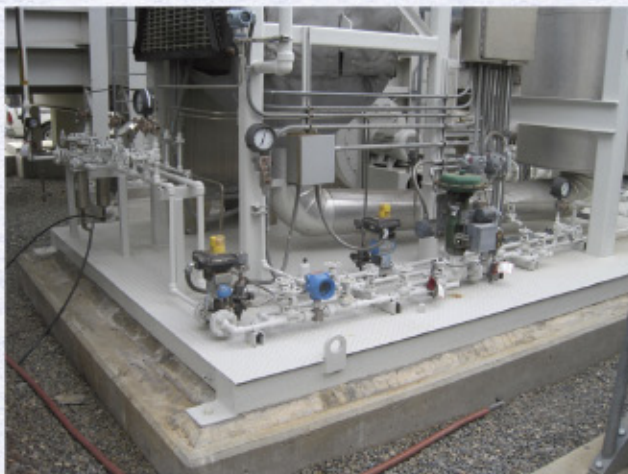
An aqua ammonia pump system for selective catalytic reduction at a combustion turbine facility.
